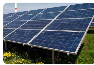
Solar panels for energy supply
